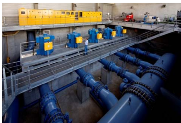
Usine de Joinville ©InnerFrance
